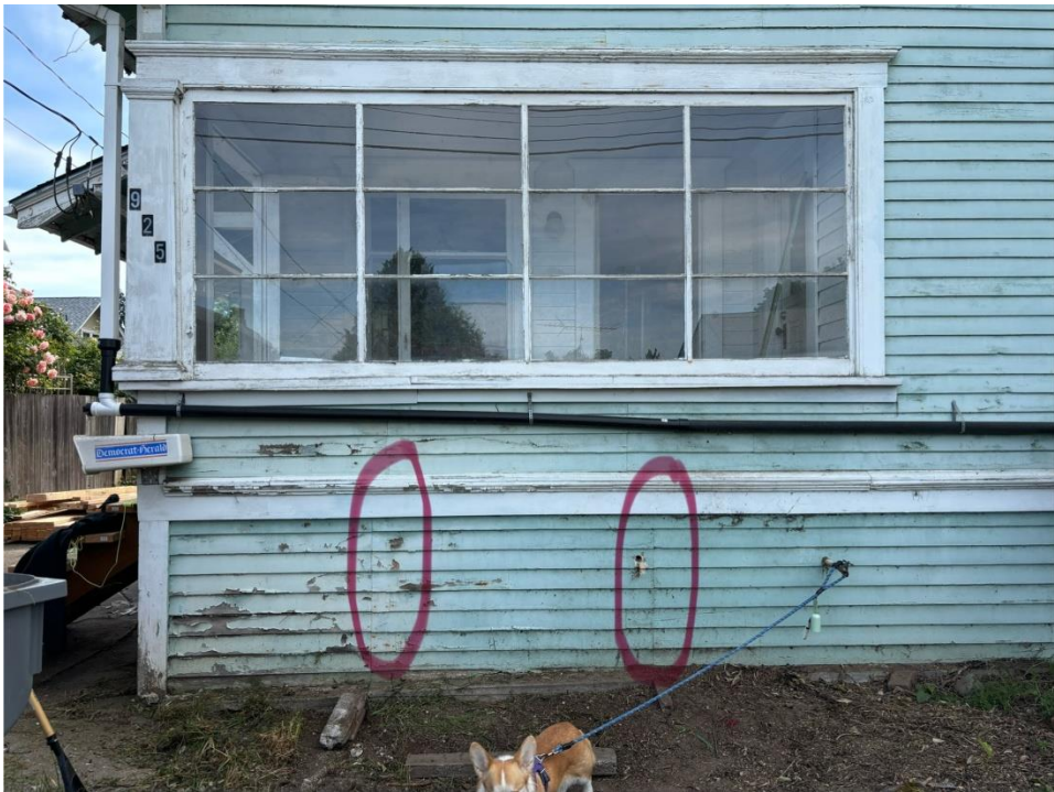
Evidence of step removal
