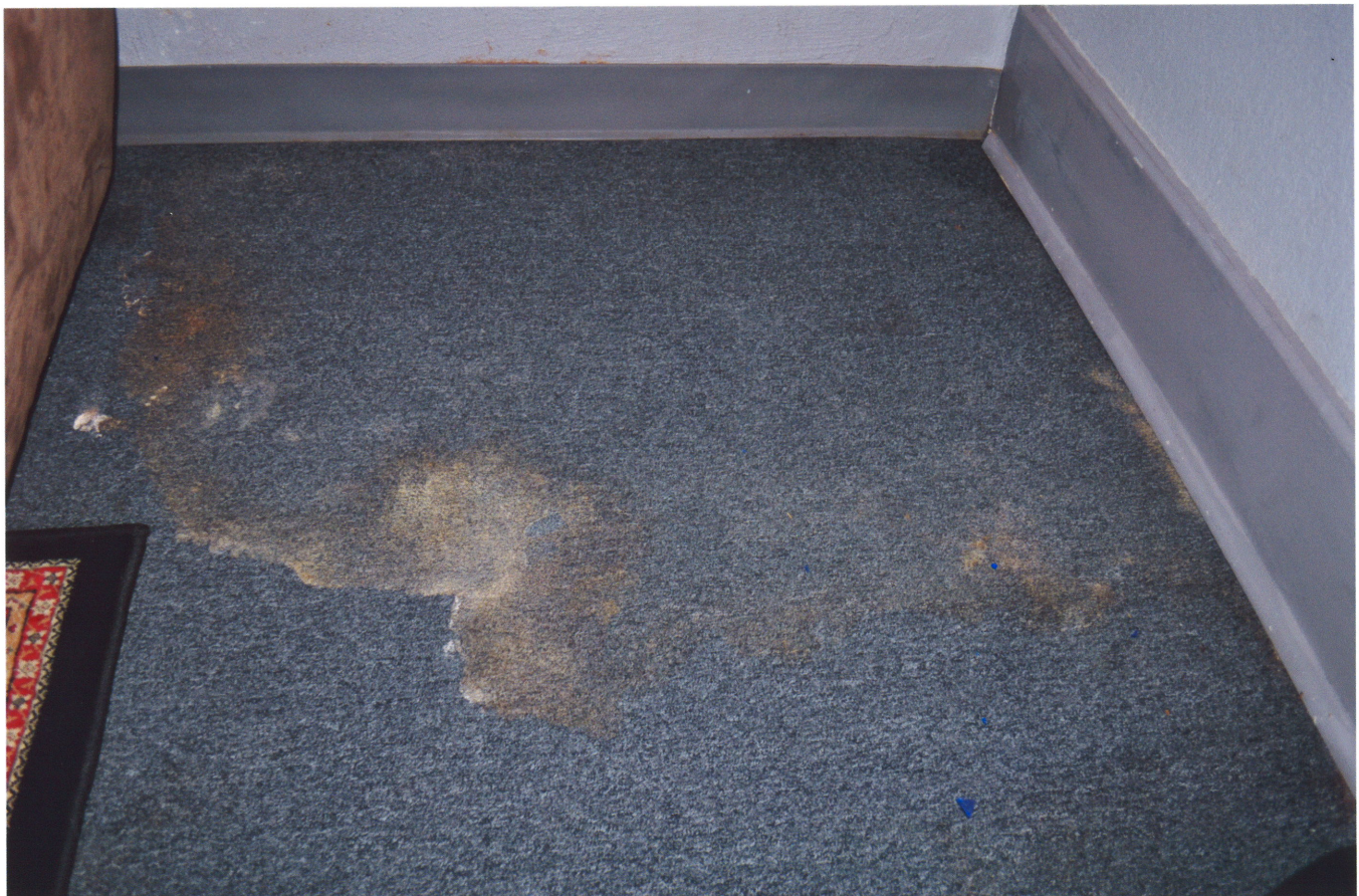
Indoor picture showing water and mold damage to carpet
