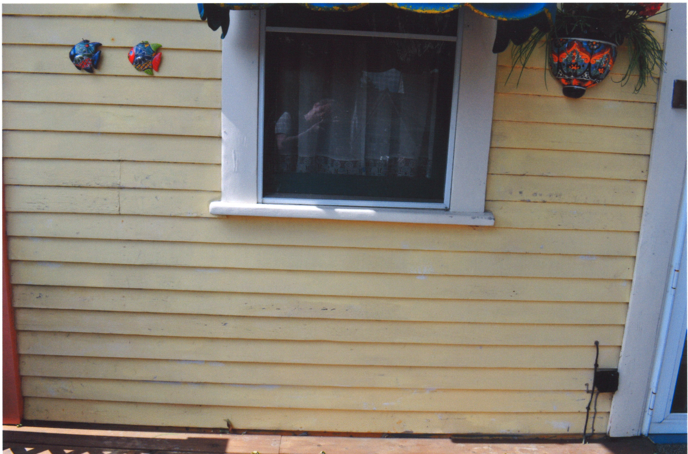
Close-up of deck area South Wall showing paint peeling off
