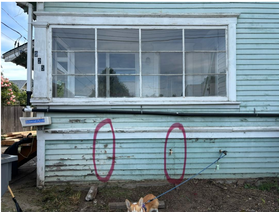
Evidence of step removal
