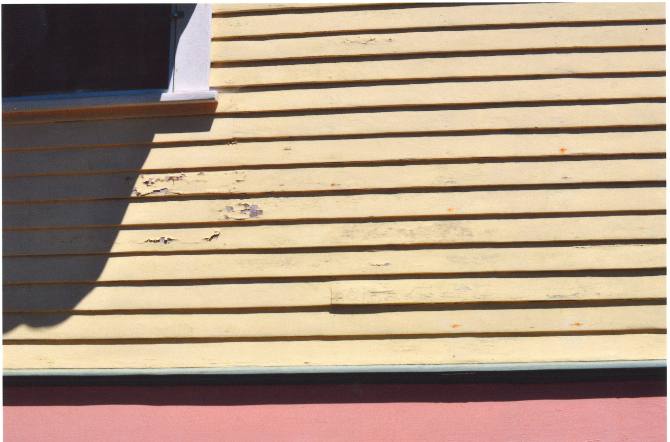
Close-up of lower right West Wall showing paint peeling off
