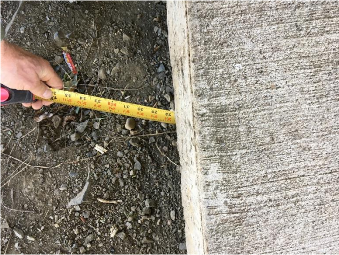
End of Lyon Street, overlook undermining, 28" lateral
