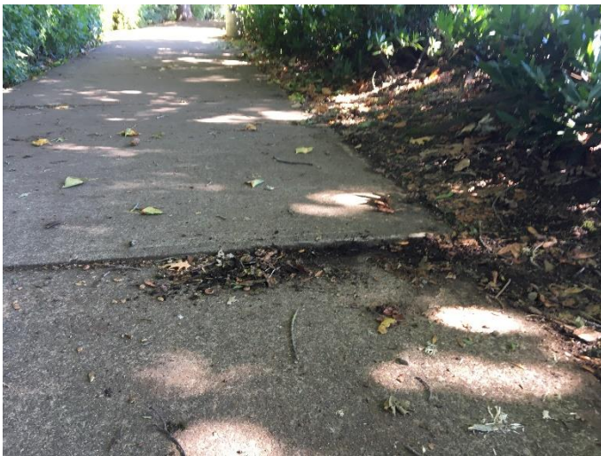
Between Ferry & Broadalbin, slab panel tilt towards slope
