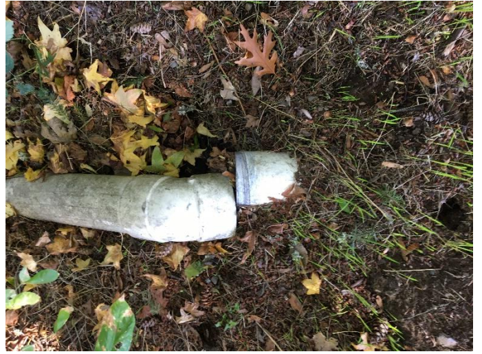
End of Ferry Street, drain pipe offset
