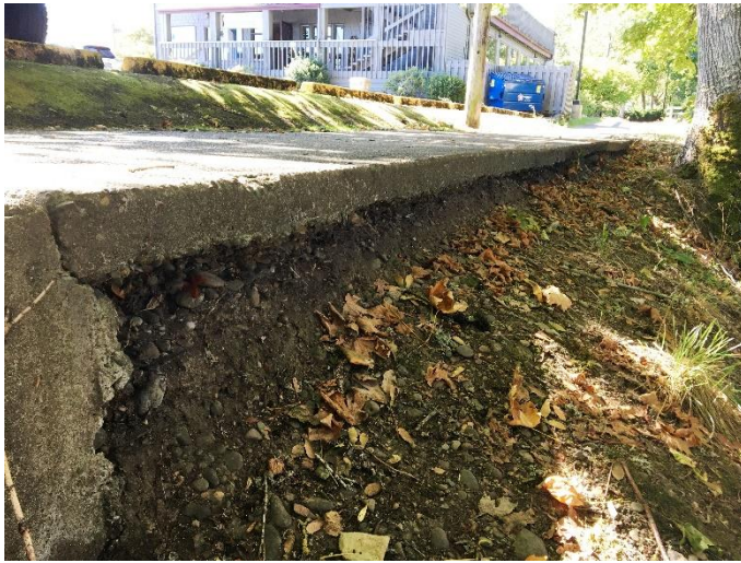
Between Broadalbin & Ellsworth, trail undermining, 9" lateral
