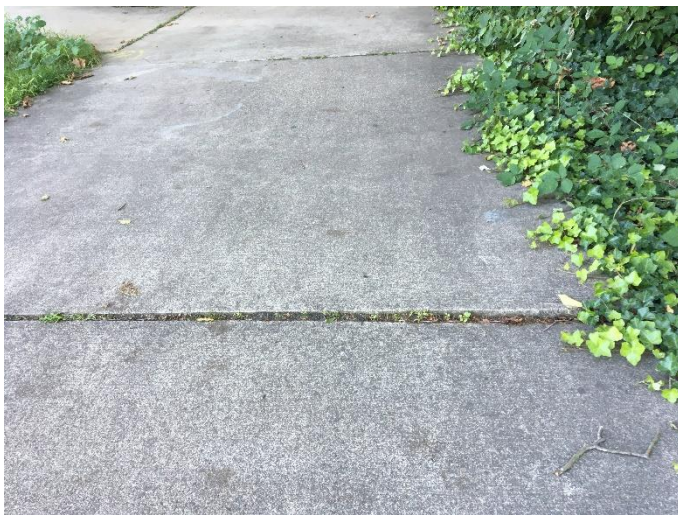
Between Ellsworth & Lyon, slab tilt towards slope
