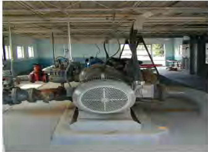
Photograph 3-2: High Service Pump Station
