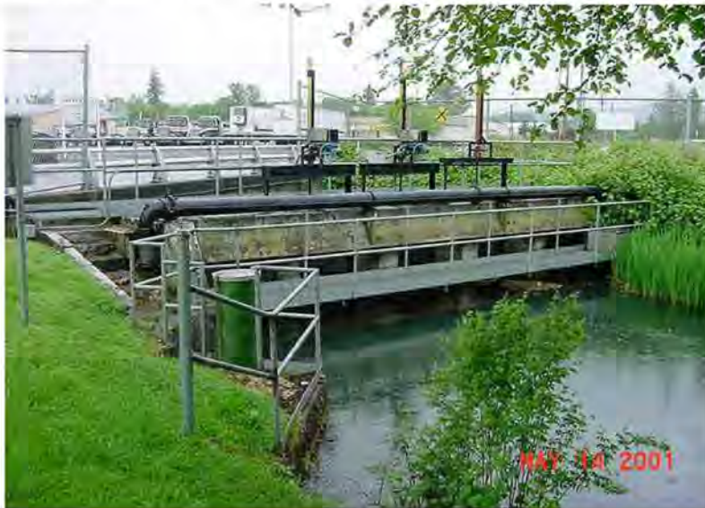
Photograph 7-11: Upstream Side of CZ Gates.
