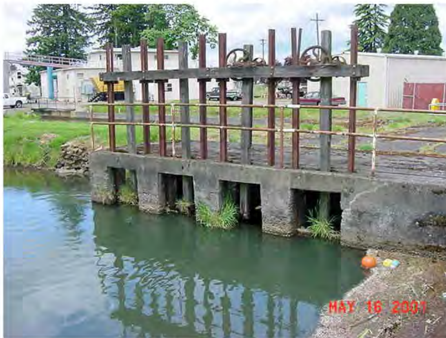
Photograph 7-9: Non-Operational Sluice Gates (Looking upstream)
