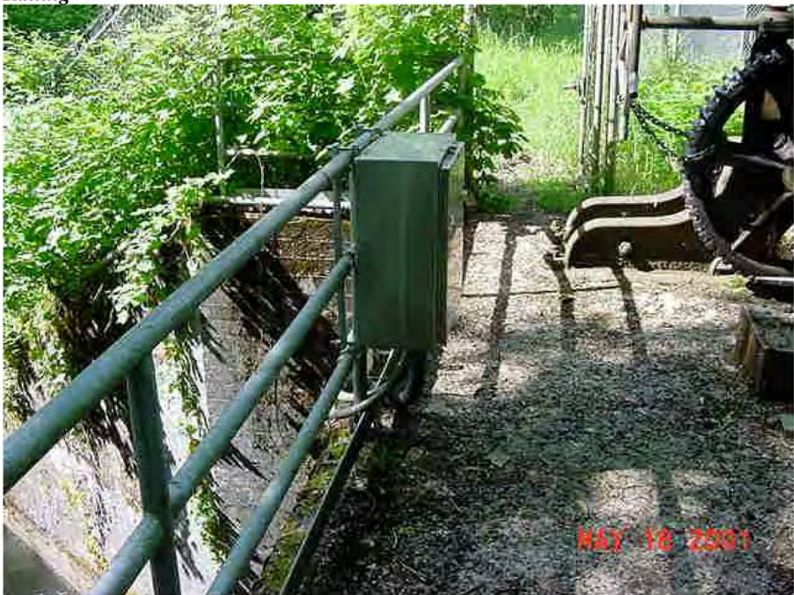
Photograph 7-5: View of Canal Headgates Remote Sensor Control Box on Deck Railing
