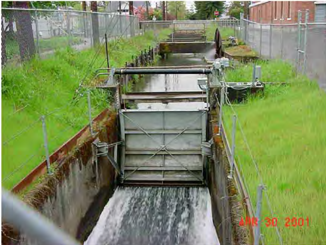
Photograph 7-20: Radial Gate at Albany WTP, Looking Upstream
