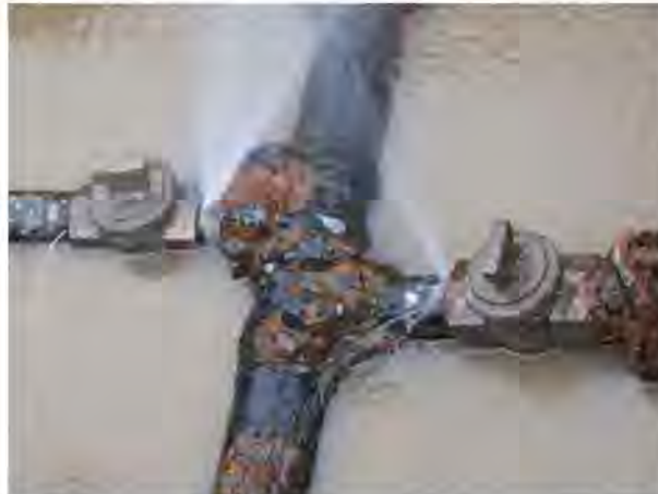
Photograph 3-1: Deteriorating Steel Water Line
