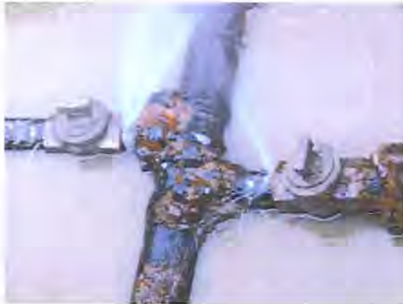
Photograph 1-1: Deteriorating Steel Water Line
