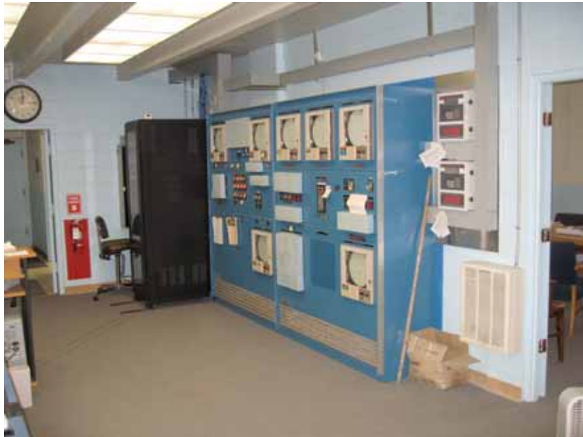
Figure 5-3. Floor Standing Cabinets
