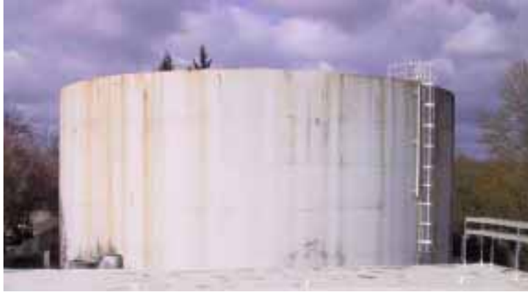
Figure 2-10. Maple Street Tank
