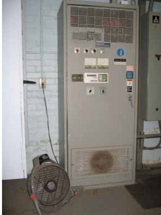
Figure 5-5. Control Cabinet for Pumps (Unanchored)
