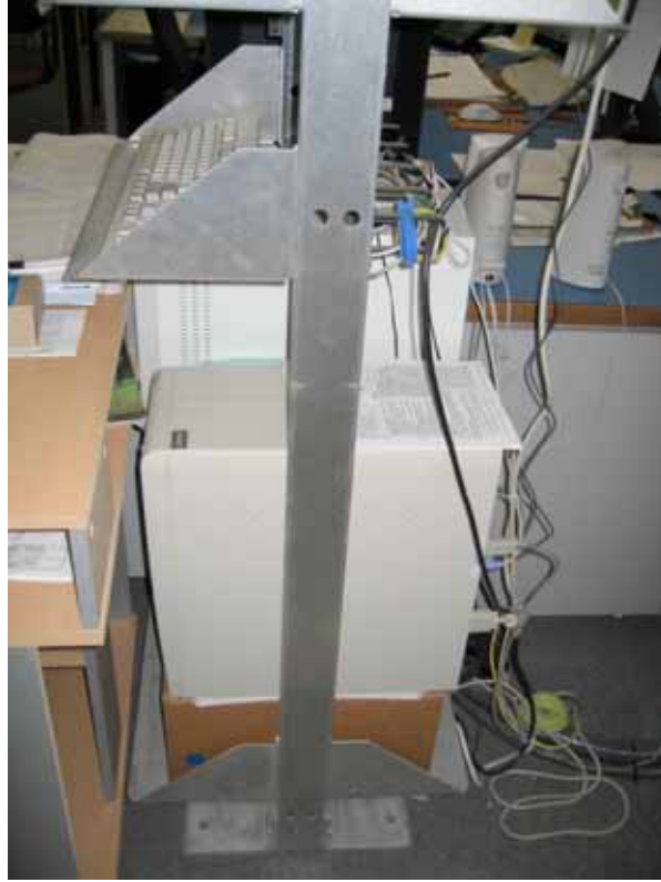
Figure 5-2. Unanchored Equipment Rack
