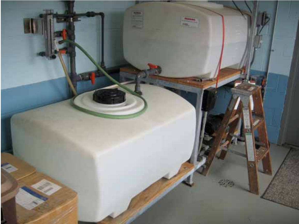
Figure 5-10. Poorly Restrained Chemical Tanks
