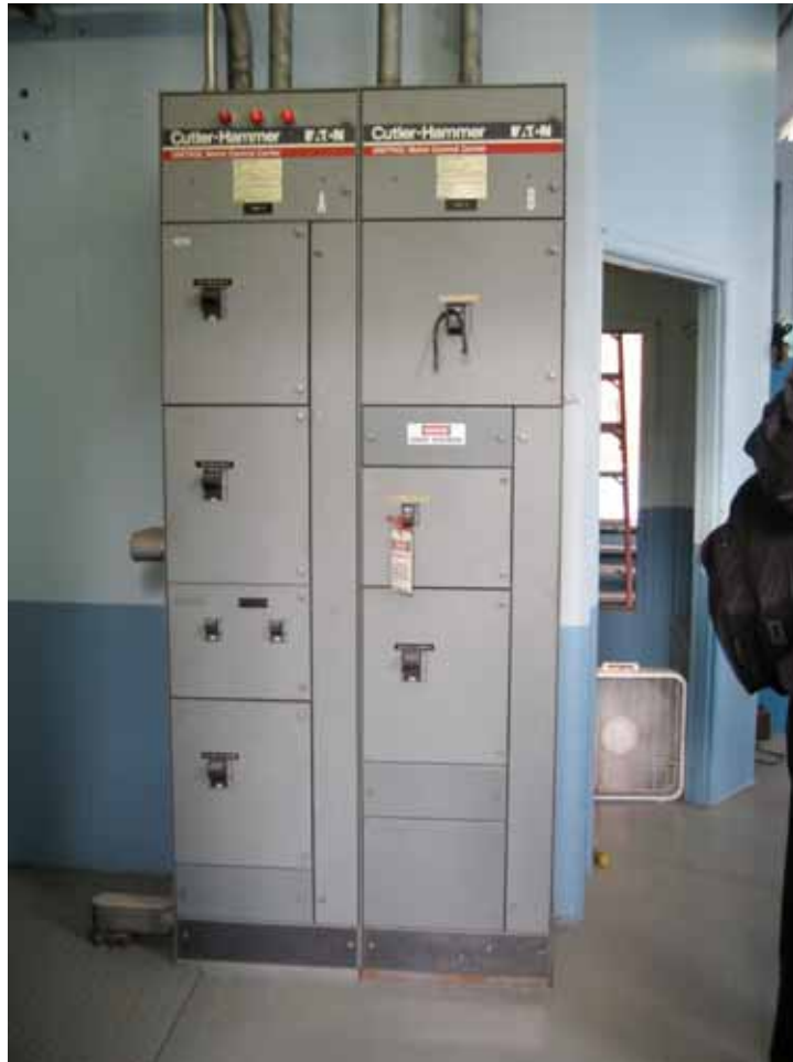
Figure 5-8. Restrained Control Cabinet
