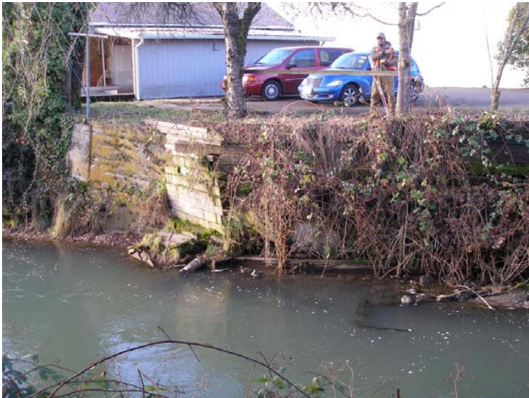
Figure 25: Failed retaining wall in Lebanon near station 771+45
