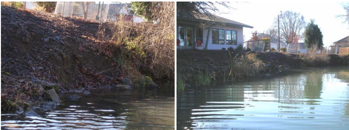
Figure 22: Bend scour present near station 702+60
