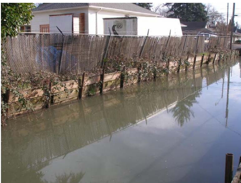
Figure 26: Inadequate Retaining Wall in Albany Station 3+38
