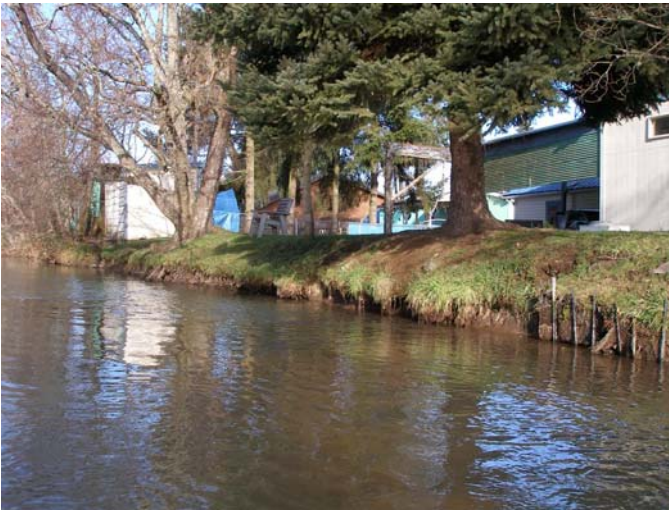
Figure 23: Bank slough failure near station 797+13
