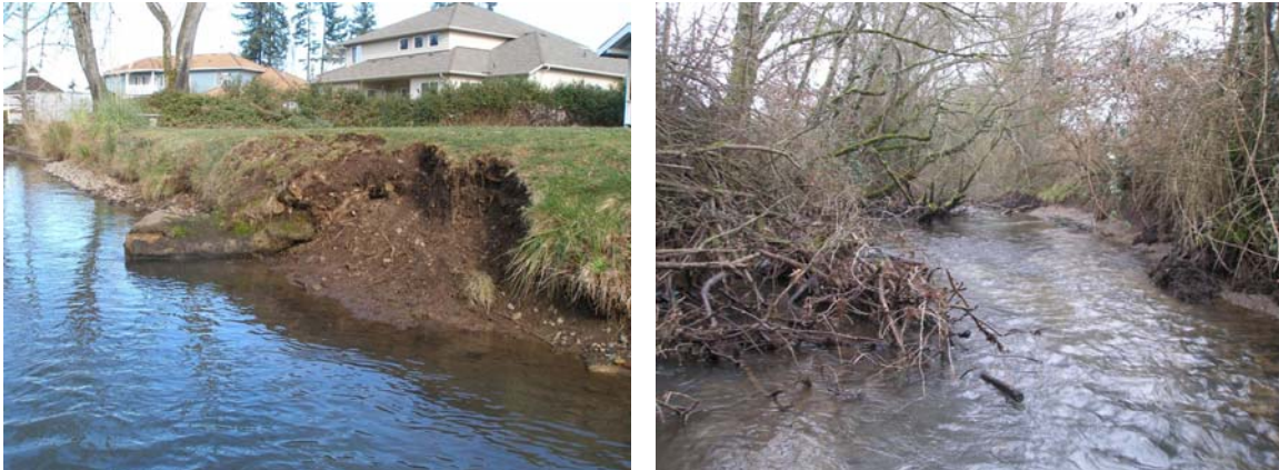
Figure 21: Examples of Impinging Flow and Back Eddy Failure Mechanisms
