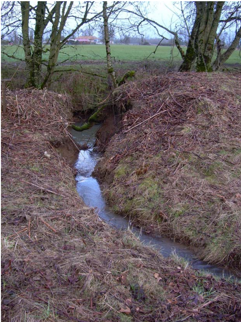
Figure 15: Overland Flow Gullying Downstream of Cox Creek Crossing 426+00
