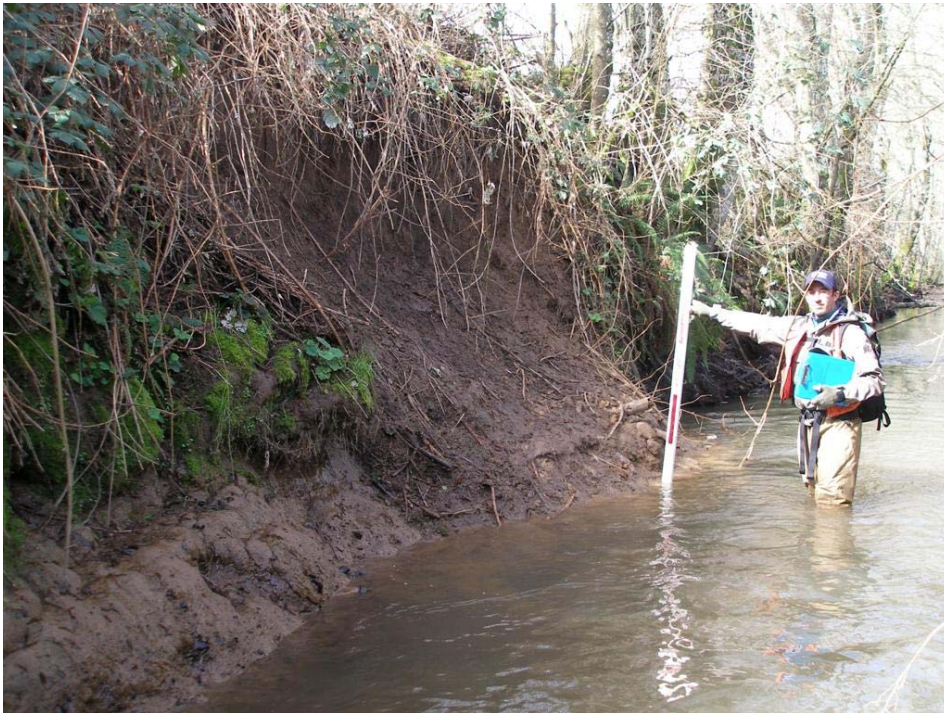
Figure 14: Saturated Soils Leading to Bank Failure Near Station 340+00
