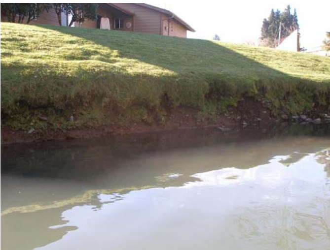
Figure 24: Bank slough failure near station 724+62
