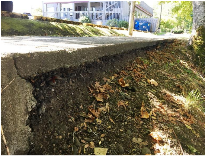
Between Broadalbin & Ellsworth, trail undermining, 9" lateral
