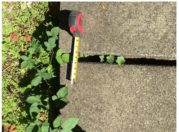
Between Ellsworth & Lyon, slab panel lateral offset
