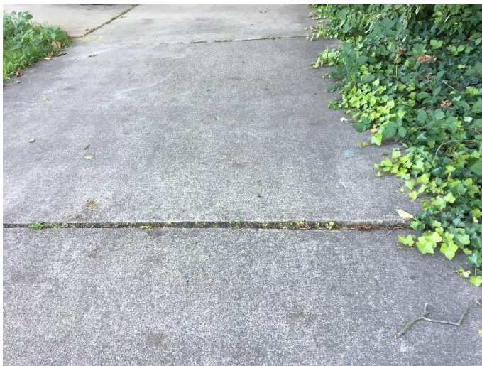
Between Ellsworth & Lyon, slab tilt towards slope
