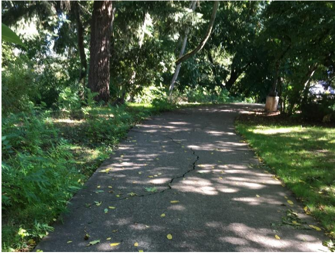
Between Washington & Ferry cracks to 3/4" width
