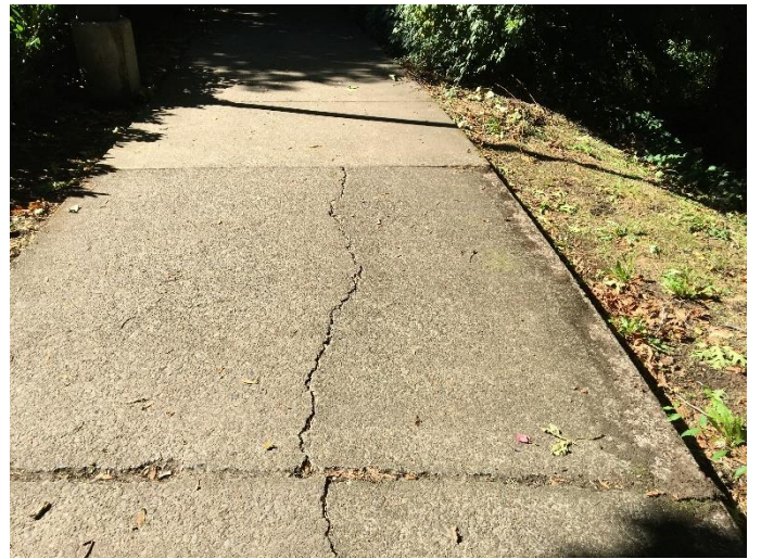
Between Ferry & Broadalbin, parallel crack & slab tilt
