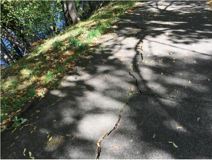
Between Lyon & Baker, cracks to 1" width
