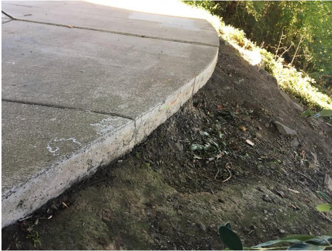
End of Lyon Street, overlook undermining, 28" lateral
