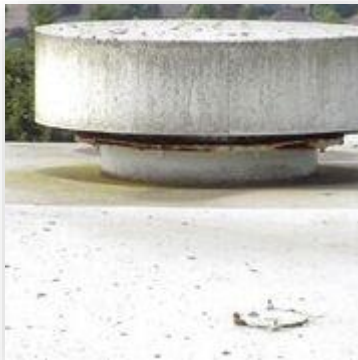
South Reservoir Vent 4
