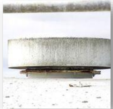
South Reservoir Vent 2
