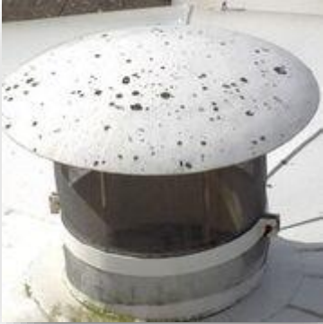
Central Reservoir Vent
