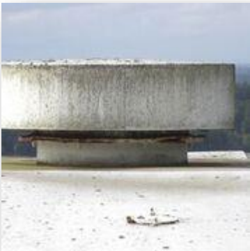
South Reservoir Vent 3
