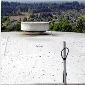
South Reservoir Vent 1
