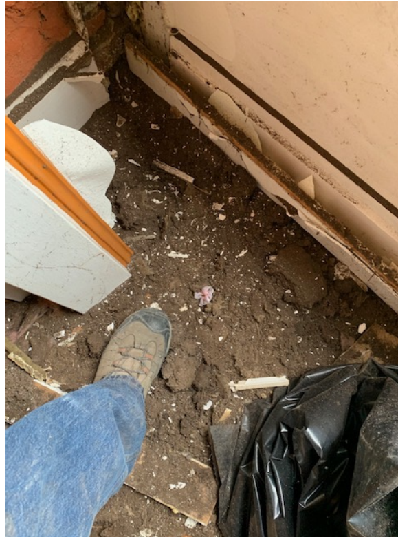
Waste on Floor Having Fallen from Ceiling
