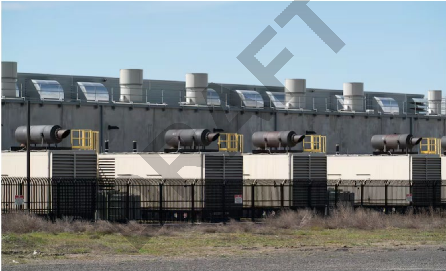
Generators and their exhaust pipes are visible outside of an Amazon data center in Umatilla, Ore., in April 2026.
