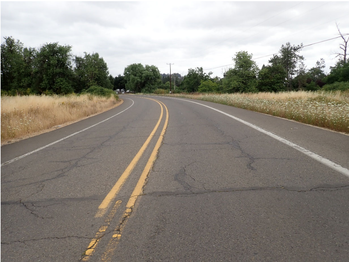
8. Looking eastbound from 450 feet east of Timber Ridge Street.
